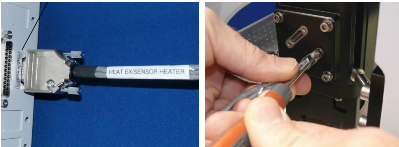
Figure 5.29: Electrical connections to the Mercury iTC
