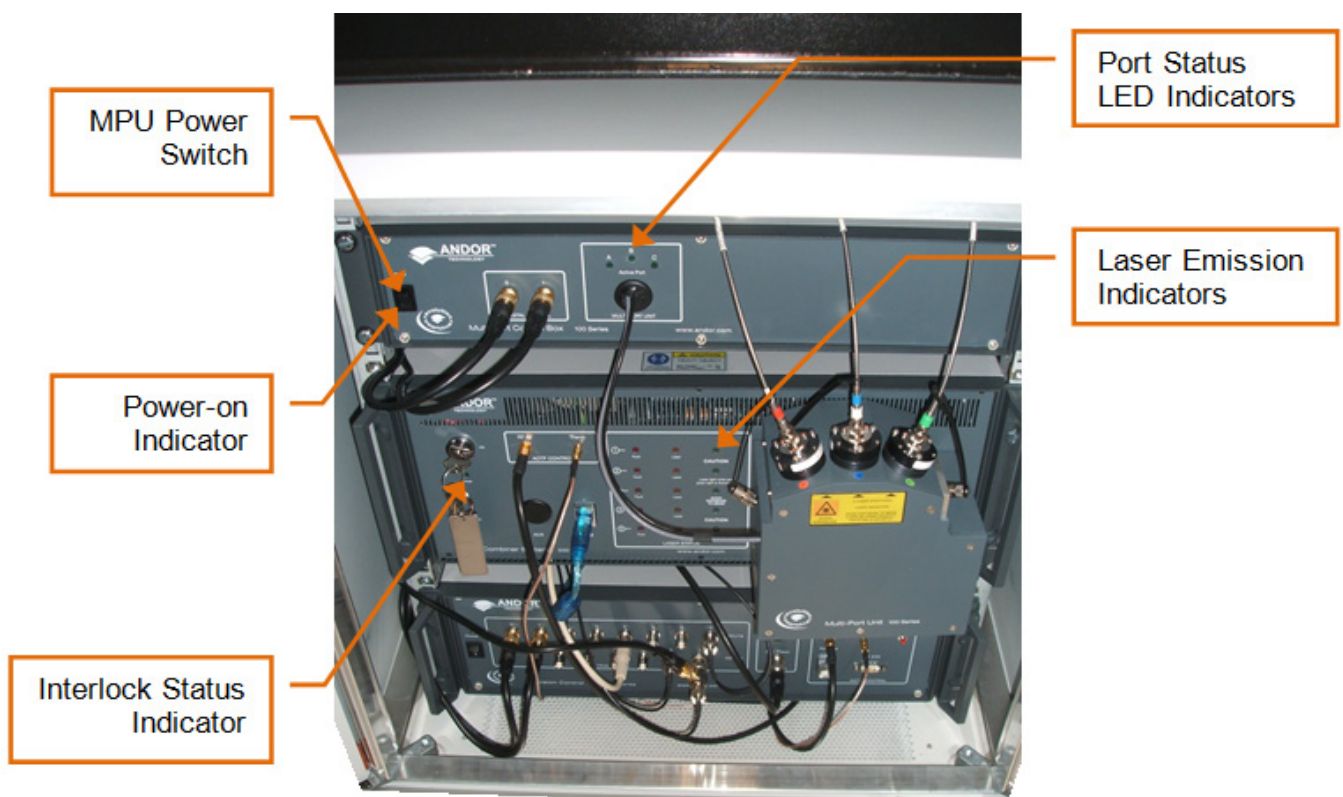
Figure 12: MPU Switch and Indicators
